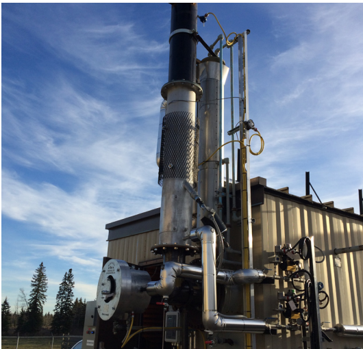
SlipStream® GTS-DeHy glycol reboiler building showing new main burner and aux burner assemblies
